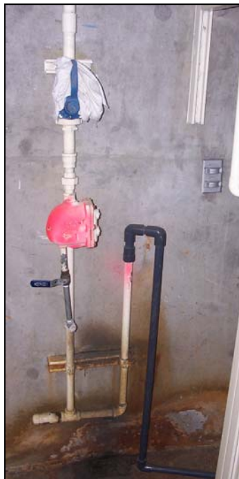
Figure 3-7. Manual drip trap modified with water seal at the WPCP
