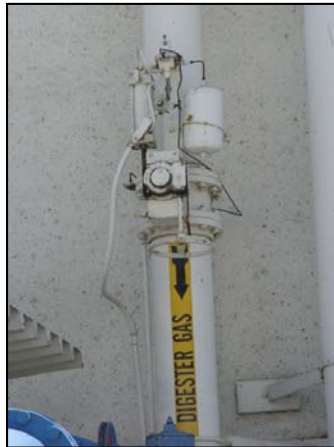
Figure 3-4. Typical emergency shutoff control valve at the WPCP
