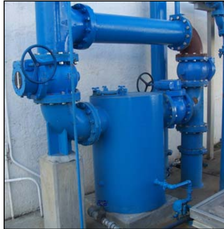
Figure 3-5. Typical sediment trap at the WPCP
