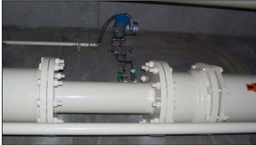
Figure 3-8. Typical digester gas flow meter at the WPCP
