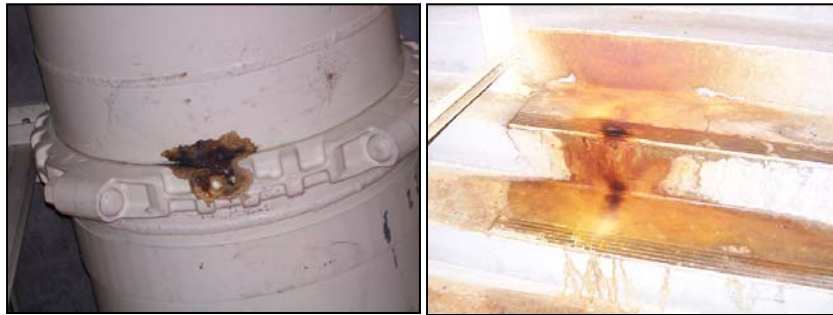
Figure 3-10. Digester gas manifold at the WPCP with a leaky joint (left) and water accumulation below (right)
