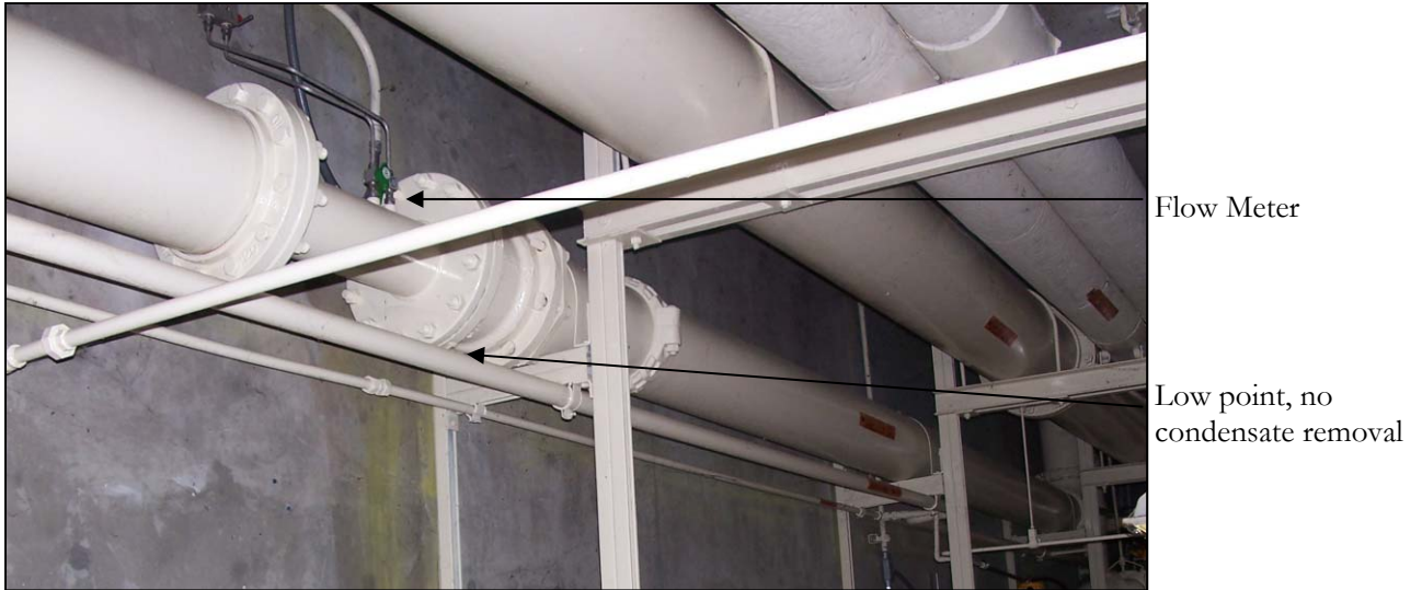
Figure 3-6. Inadequate condensation removal upstream of flow meter at the WPCP
