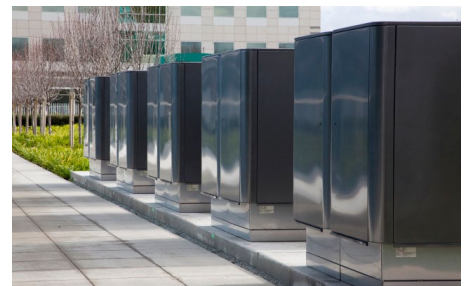
Photo: Bloom Energy Servers at eBay, San José, California.
