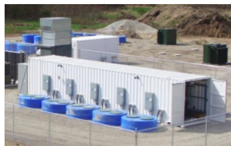
Photo: 3 MW Mechanical Storage for Ancillary Services, NE ISO (Beacon Power).
