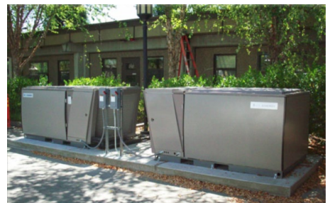
Photo: 12 kW Thermal Storage, Napa Community College (Ice Energy).
