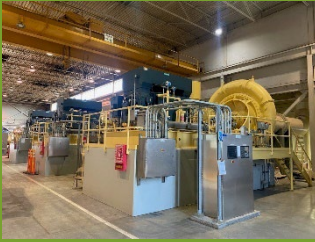
Process Air Blowers with improvements
