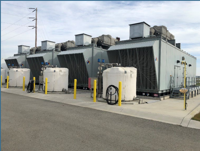
Emergency diesel generators, a key consideration in the upcoming assessment of RWF Emergency Power Strategy
