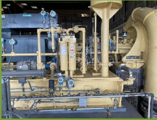
Secondary Blower with Improvements
