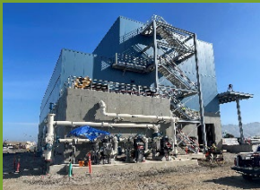
Centrate pumps at South Side of Dewatering Building
