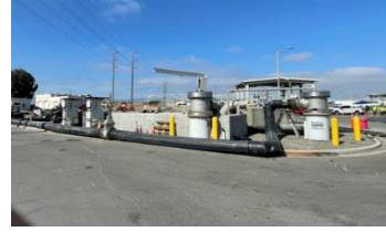
Temporary flow diversion system including reroute piping and pumps
