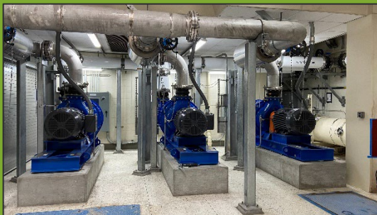
Three new Centrifugal Blowers for the new Filter Air Scour System
