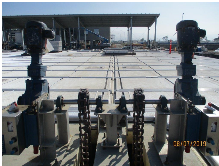
Figure 4: DAFT covers and equipment
