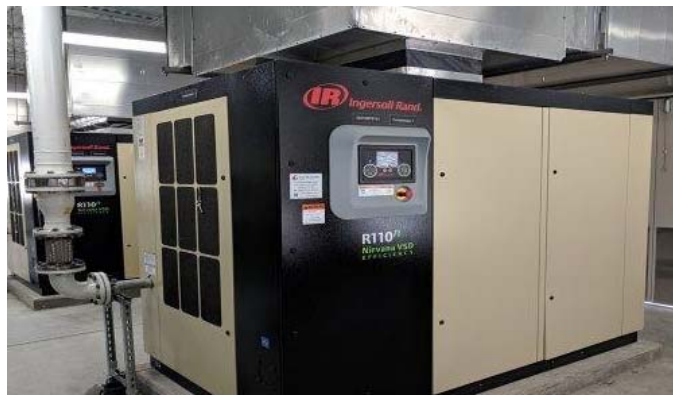
Figure 7: New Air Compressors
