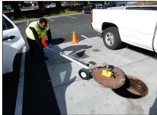
Inspector Mahmoud Jillo lifts the cover off a restaurant grease interceptor during a February 2017 inspection.
