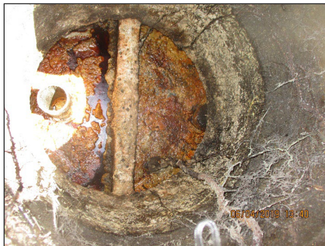
FIGURE 30. INSPECTING A COMMERCIAL GREASE INTERCEPTOR
